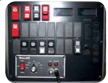
Paragon Electrical System
