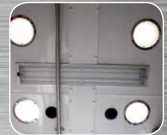
Ducted Heat/AC System
